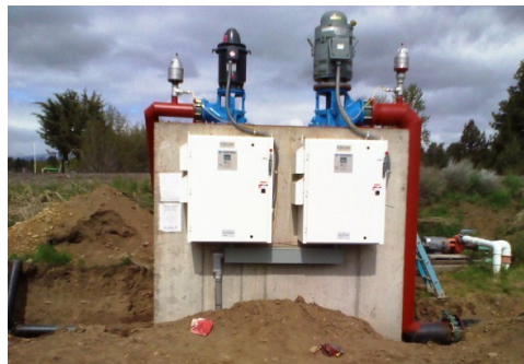
After System Improvements —White cabinets are the two Variable Frequency Drives. Two new pumps installed above the VFD’s. VFD/pump on the right services northern 26 landowners, left side services 4 southern landowners.
