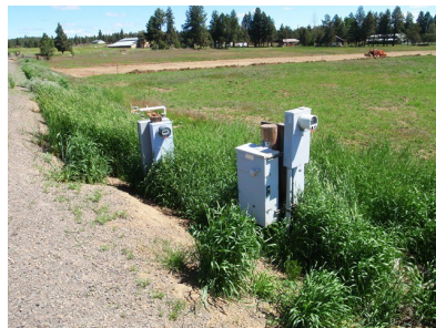
Before System Improvements —Hurtlely Ranch Road irrigation pumps and electric meters. View is facing north, pump/meter on left in photo serviced 26 landowners; right serviced four to the south.
