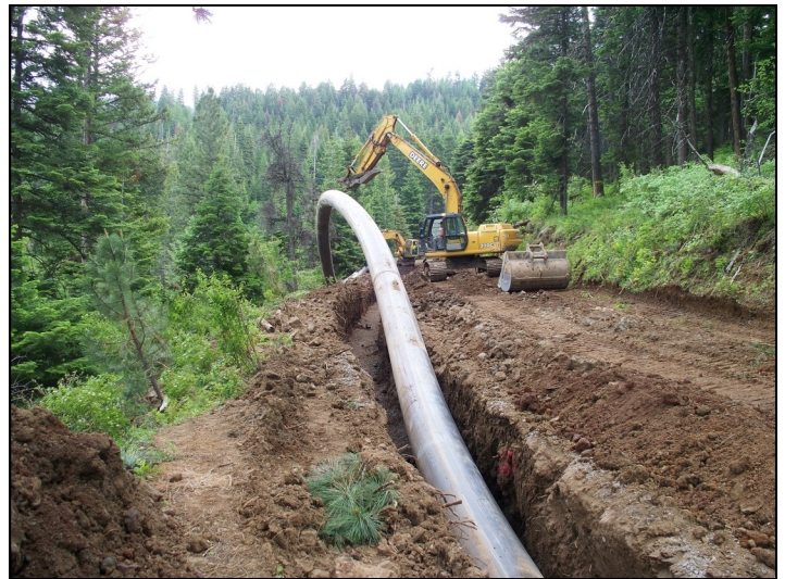
The entire 7,800 feet of HDPE pipeline for the Cove project was installed in one entire piece of pipe with no fittings. The pipeline route was on a narrow mountain right-of-way cut into a steep hillside which made installation challenging. Photo courtesy of Anderson Perry & Associates, Inc. of La Grande.
